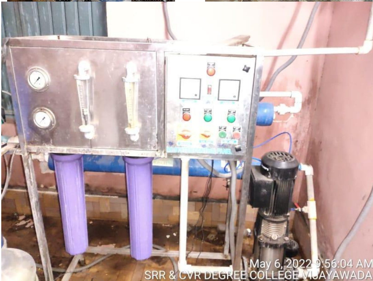
Fig:- RO Water Unit
